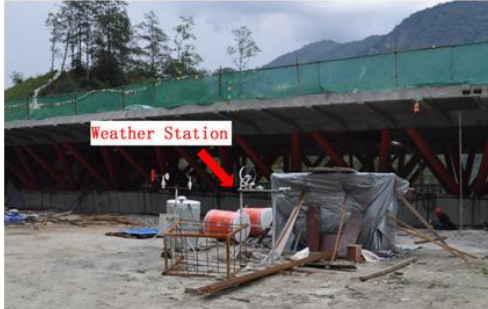
Fig. 3 Weather station in the field
