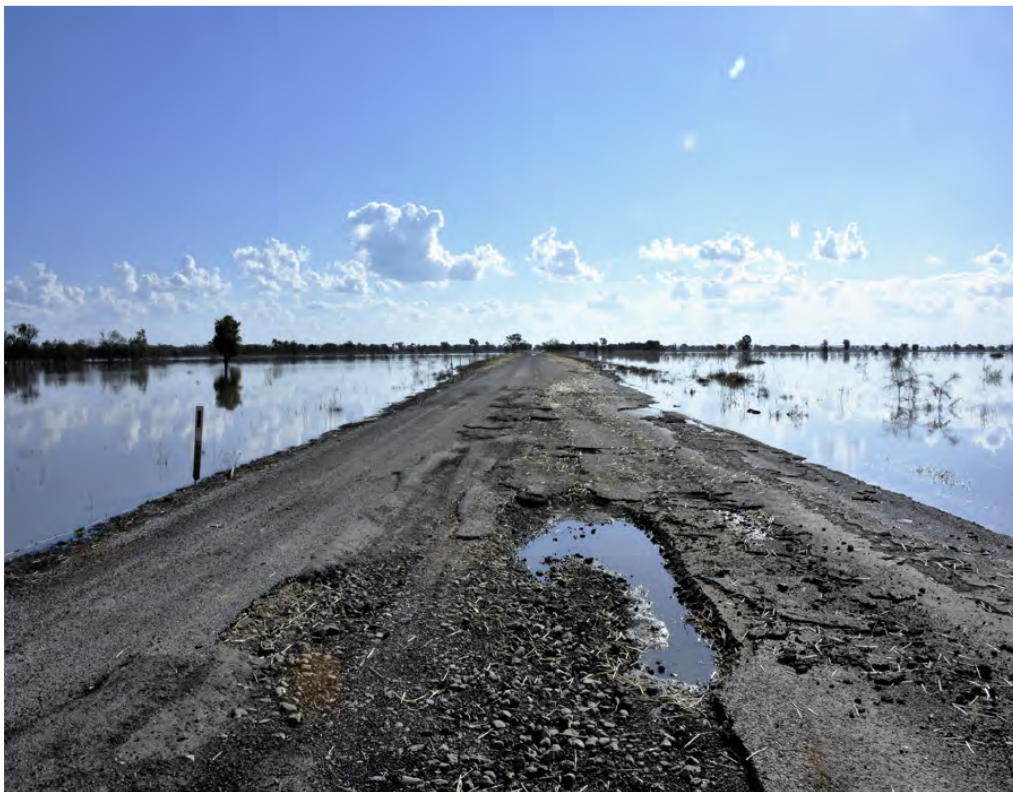
Figure 7: Flood damage to roads
