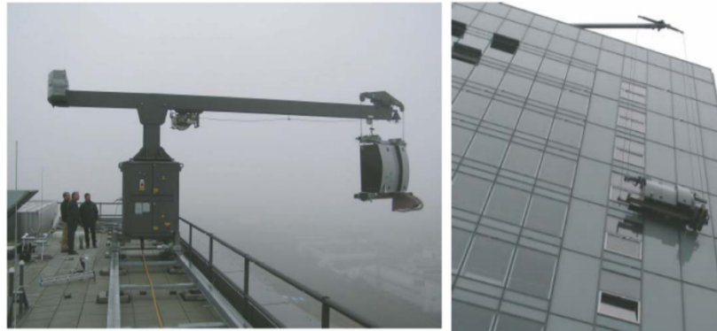
Plate 3 Rooftop Gantry of SIRIUSc (Elkman et al. 2005)
