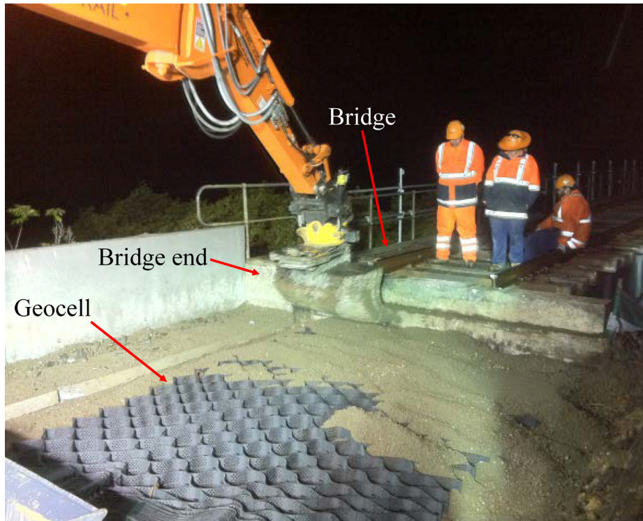
Fig. 8. Installation of geocells at the railway bridge ends on the south coast line of New South Wales, Australia (modified from [46])
