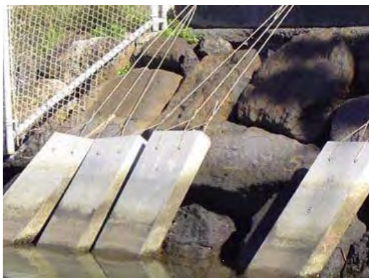
Figure 7: RC slabs exposed in Honolulu Harbor [92]
