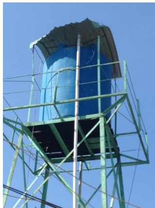
Figure 6. Private Enterprise owned and managed water tower in Region 1, Mekong Delta, Viet Nam.
