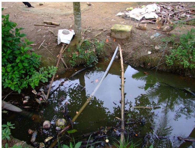
Figure 1. Private water supply pipeline crossing a water course in Region 1 - rural Viet Nam
