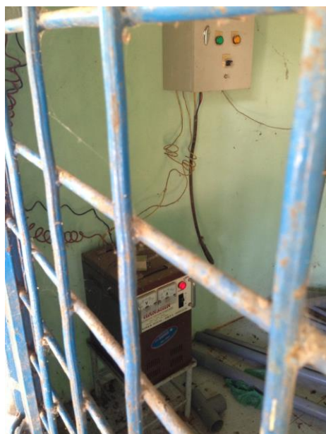
Figure 69. Inside the Song Thu pumping station
