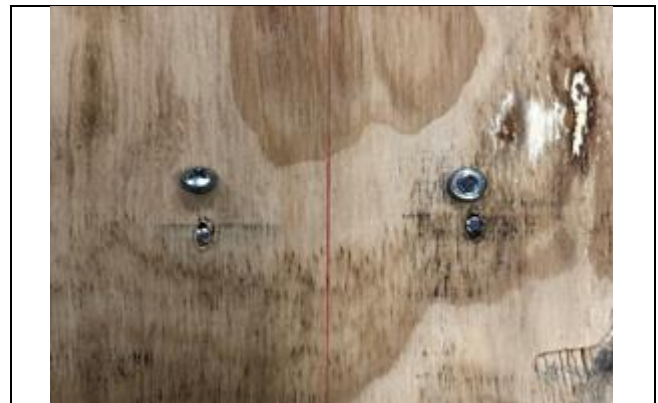
(a) Shear failure under the head of the screw
