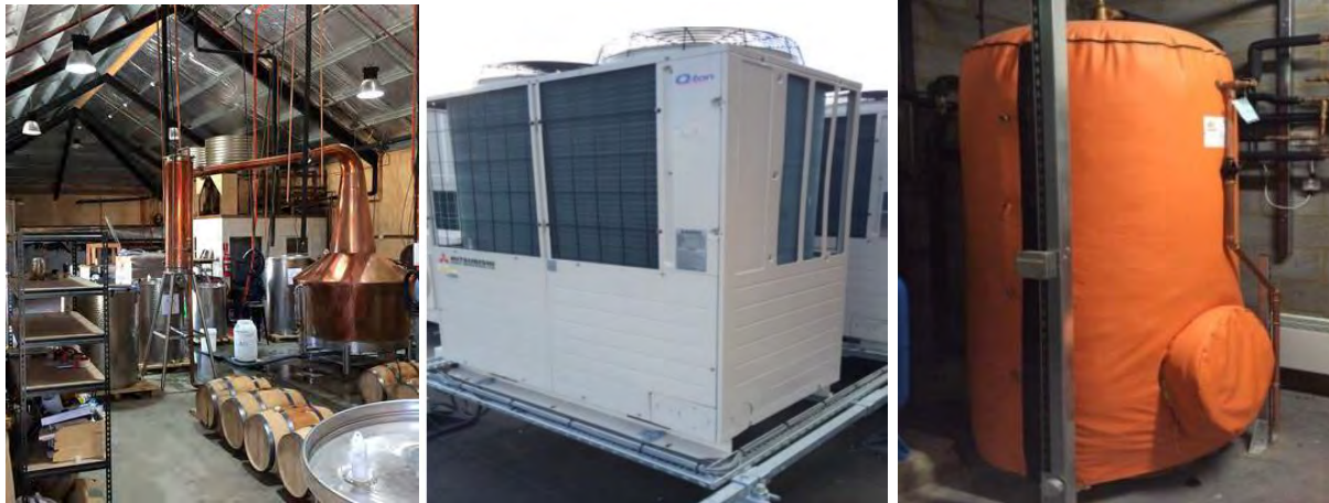
Figure 46: Left: Shene Estate and Distillery, TAS; Centre: Example of a Mitsubishi Q-ton unit; Right: hot water storage tank coupled to Q-ton unit. (Reproduced from Mitsubishi Heavy Industries).
