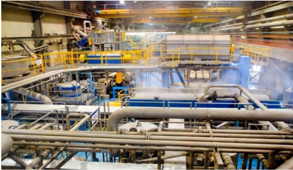
Figure 65. Visy's waste to energy plant in Coolaroo, VIC. (Reproduced from protechwelding.com.au .)
