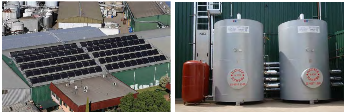
Figure 44: Evacuated tube collectors and storage tanks. (images from Apricus).
