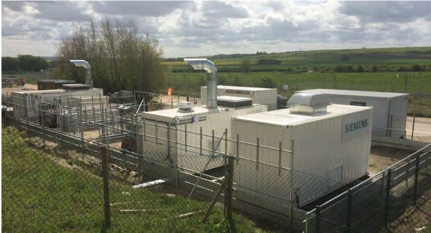
Figure 51: Siemens green ammonia pilot project at Rutherford Appleton Laboratory, near Oxford, UK. (Image from ammoniaindustry.com.)
