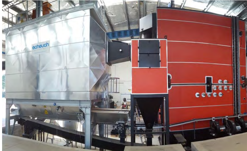
Figure 69: Biomass boiler (right) with exhaust gas treatment system (left). (Reproduced from Justsen Pacific.)
