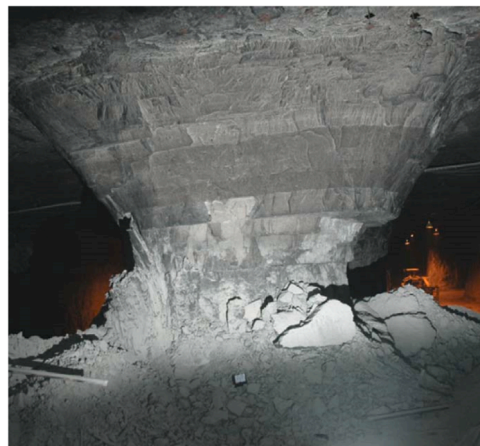
Fig. 2. Pillar that had an original width-to-height ratio of 1.7 failed by progressive spelling [28].
