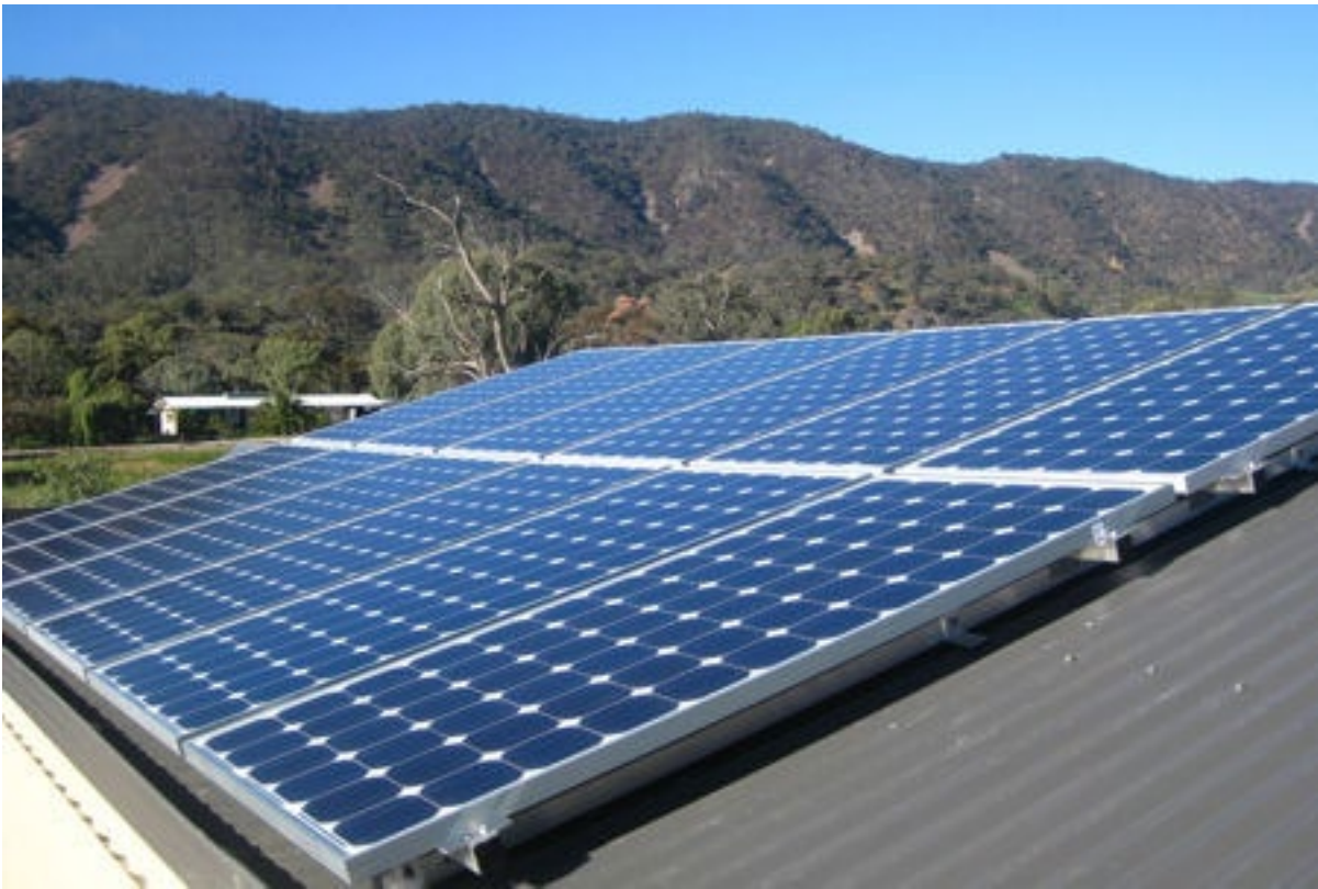
Figure 19: Small-scale rooftop solar installation
