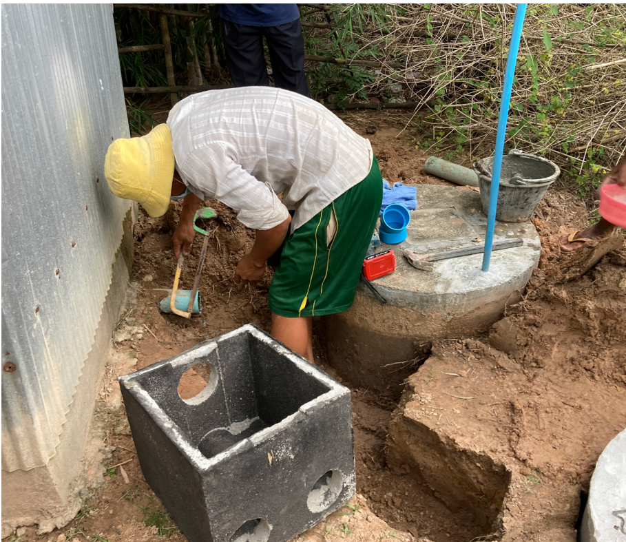
Local suppliers and masons install a twin pit latrine designed by EMW in Cambodia Credit: Thrive / EMW
