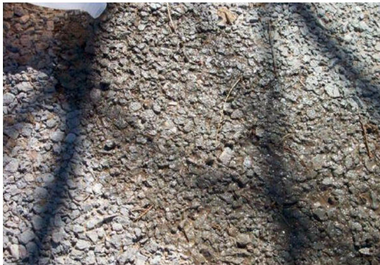
Figure 2.22 Pervious concrete clogging [2]
