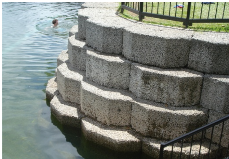
Figure 2.21 Pervious concrete blocks in Lake Eacham (Northern Queensland)
