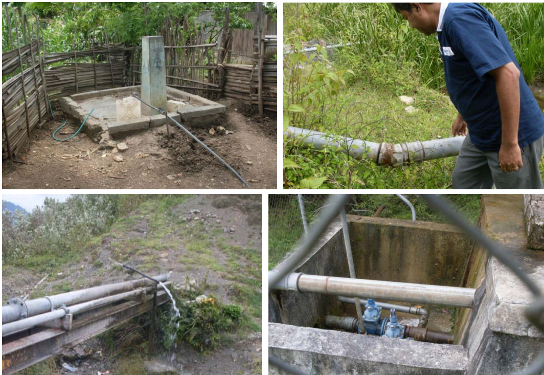
Figure 3: Common functionality problems viewed in Maliana and Atabae (Top left: unused water point due to solar pump failure, Top right: rusting pipe joint, Bottom left: mainline pipe leakage, Bottom right: leakage at intake)
