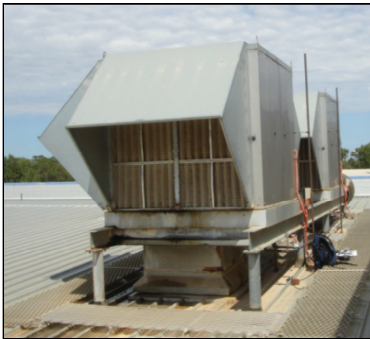
Figure 9: Large commercial direct EAC. Source: AIRAH 2010c
