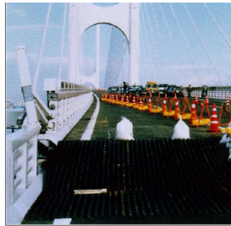
Figure 7-9 (a) Bridge configuration at 60 seconds (after earthquake) and (b) uplift of the deck around the pin-support, Higashi-Kobe Bridge after 1995 Kobe Earthquake.
