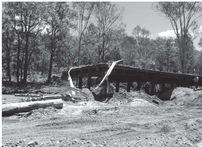
Figure 1-1 Timber bridge damaged by floodwaters (Pritchard, 2013).
