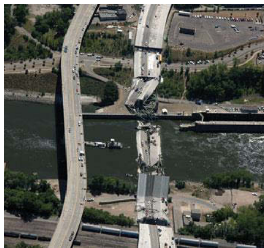
Figure 1-3 I-35W Mississippi River bridge collapse.
