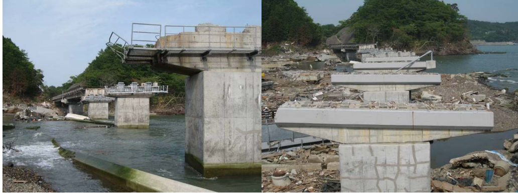
Figure 1-2 Bridges damaged by tsunami (Unjoh, 2012).
