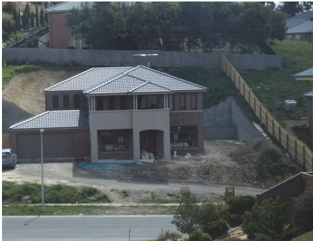
Figure 1: Example of a new residence under construction on a steeply sloping site (Note: Photograph attributed to Alistair Woodard)
