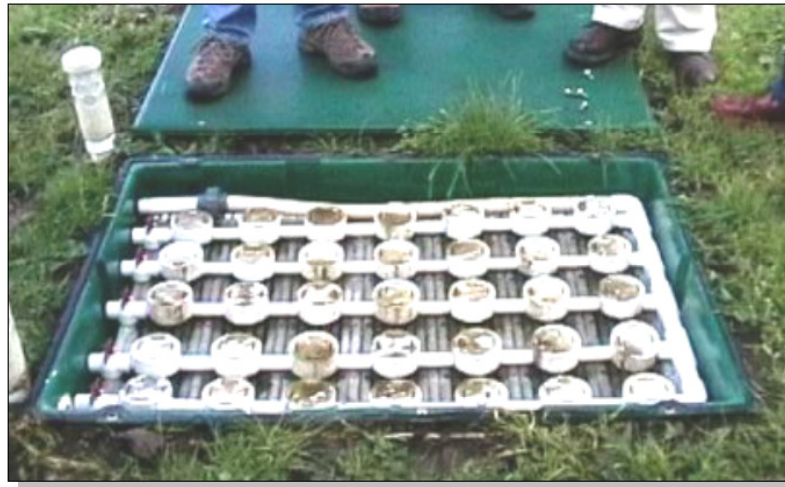
Figure 15: An installed AdvanTex system in New Zealand.
