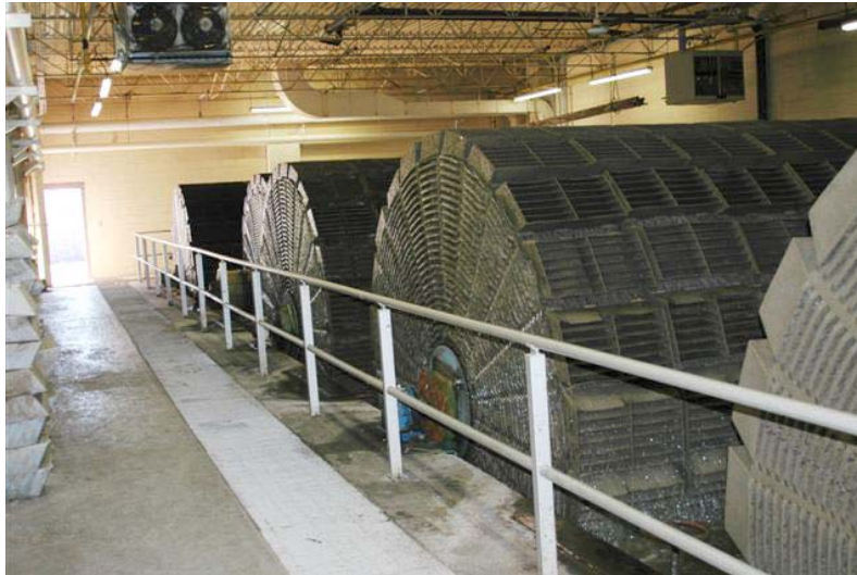
Figure 4-4 Rotating Biological Contactors (Mission Green Canada, 2006)
