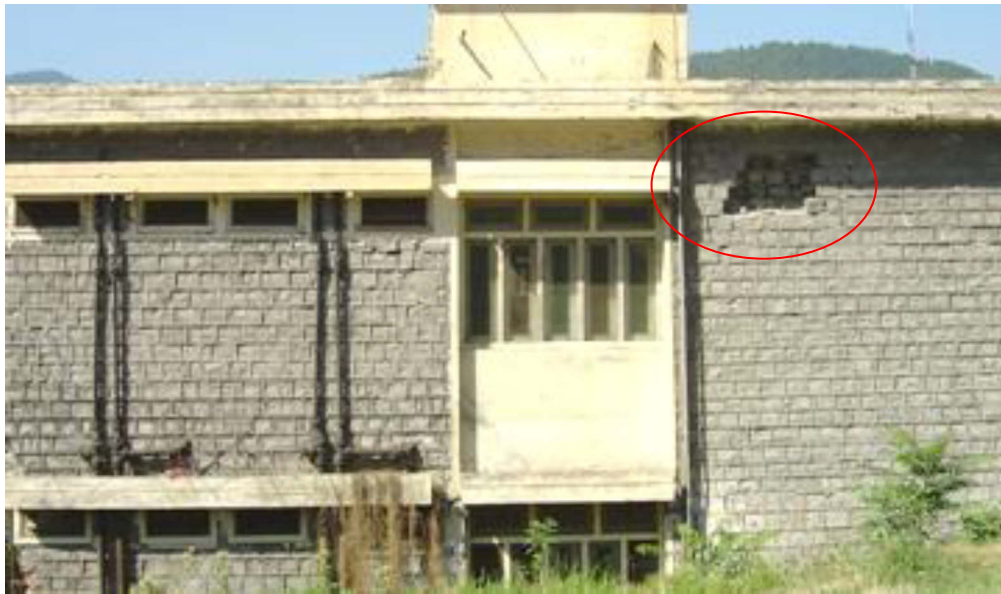
Figure 3.6 Localised damage of a wall during a seismic event ( Photo: NSET )
