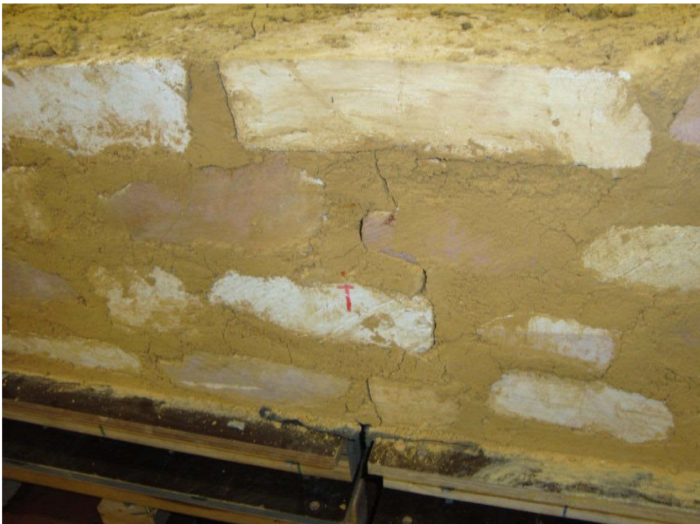
Figure 5.42 Cracks in unreinforced wall (Bending in lateral span)
