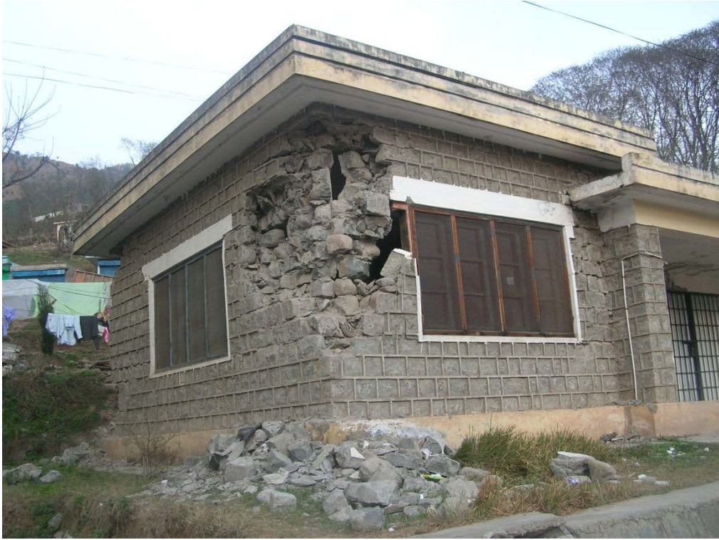
Figure 2.11 Damage along the corner ( Photo NSET )
