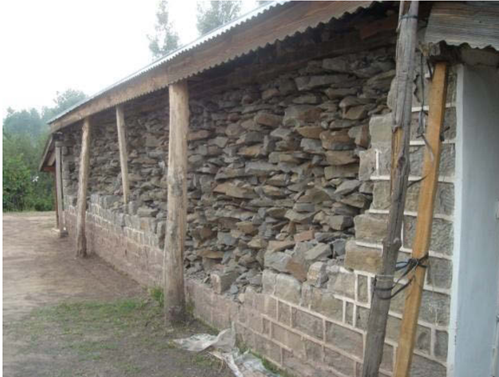
Figure 2.8 De-lamination of stone masonry (Photo: NSET)
