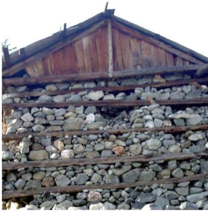
Figure 2.25 Partial damage of rubble wall with wooden bands in an earthquake
