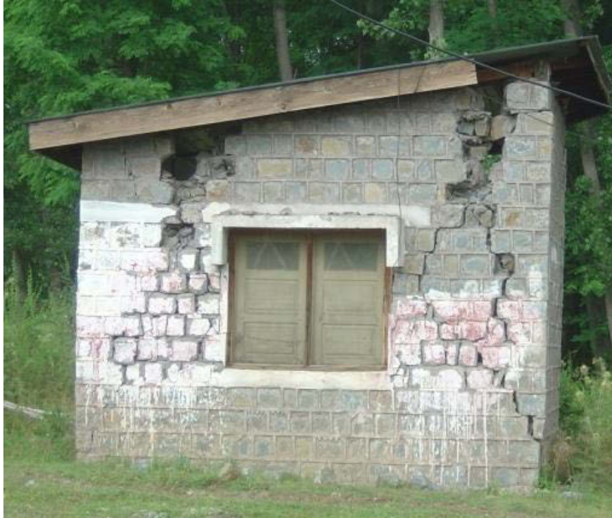
Figure 2.10 In-plane shear failure and corner separation
