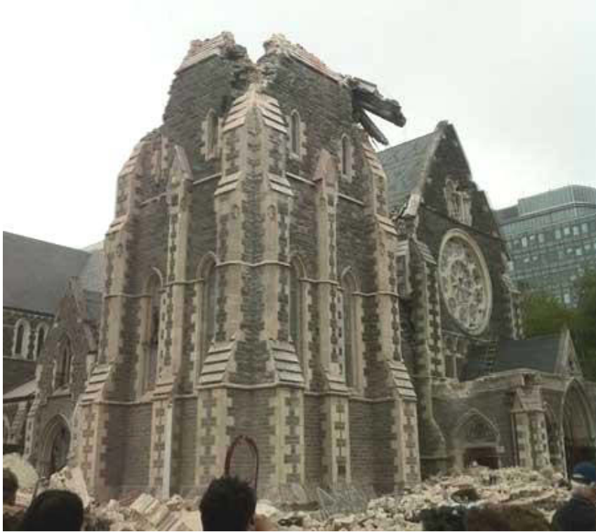
Figure 1.3 Damaged Cathedral in Christchurch Earthquake (Stuff 2011)
