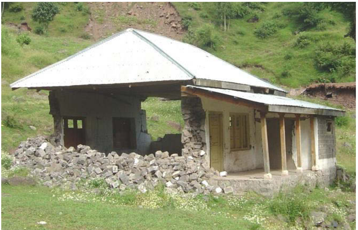
Figure 2.9 Out of plane bending failure
