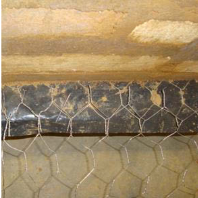
(a) Inserted nail in the middle of untwisted sides of overlapped mesh
