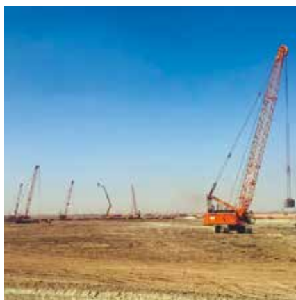
Al Zour refinery KUWAIT
