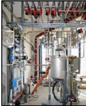
Plate 4 BIQ plant room
