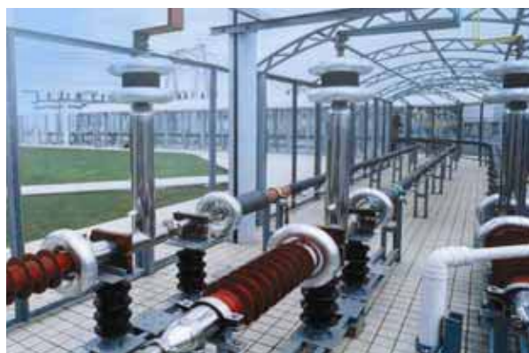
Figure 1 HTS cable site at Puji substation in China
