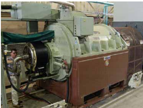
Fig. 2. 5 MW motor coupled to two 2.5 MW load motors at CAPS [6].
